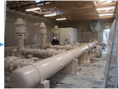
7 Pump Stations (5 Pressure Zones)
