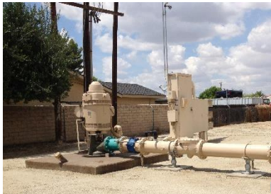
Groundwater 6 Active Wells (10 total)
